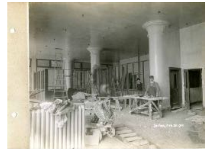
Ford Building, interior photo, 1914. Note the ornate capitals atop the columns. Photo courtesy Brian McMahon
